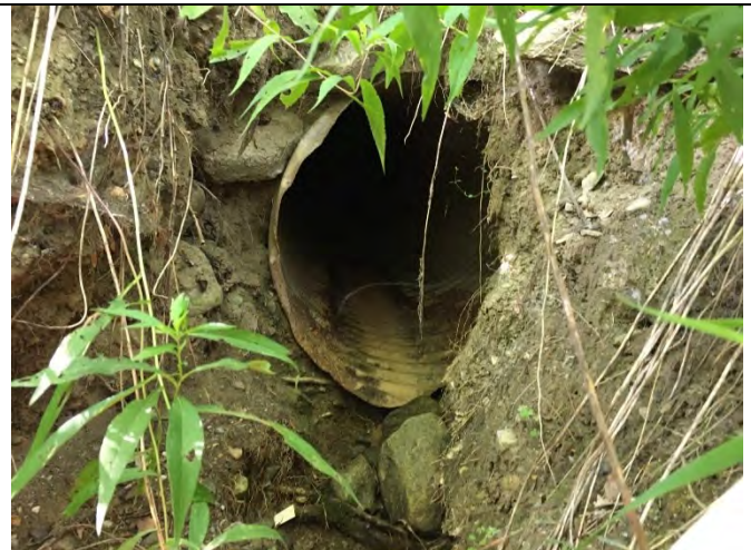
Photo 2: Outfall from the system with gully erosion into stream.
