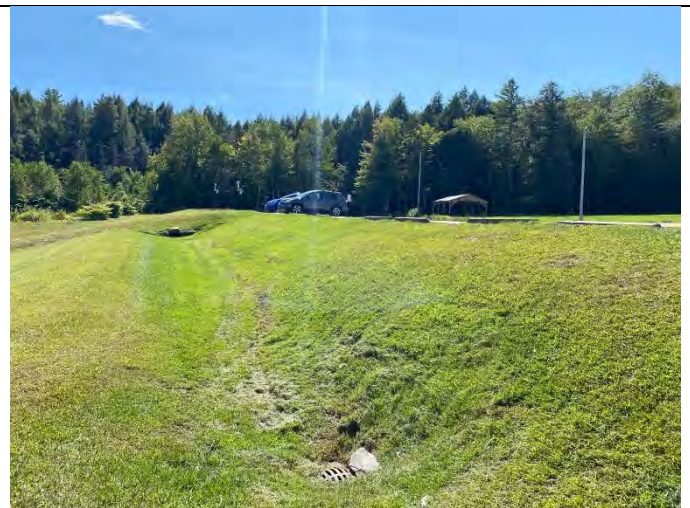
Photo 2: Swale along east side of parking lot that does not receive runoff due to poor site grading
