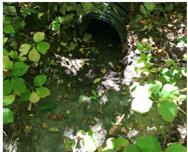
Photo 2: Sediment deposition at the outlet of the culvert.
