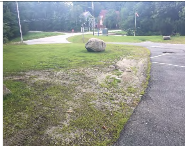
Photo 1: Sediment deposition at low point of the parking lot where water runs off. Ineffective catch basin in the top right corner.
