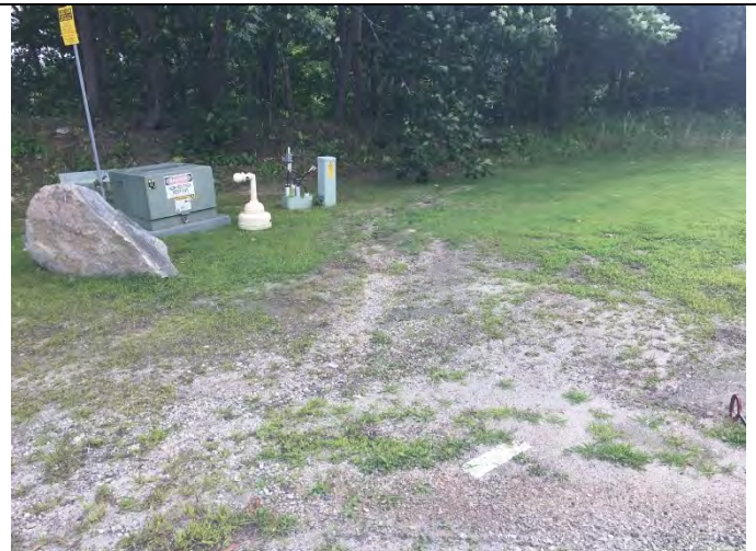
Photo 2: Minor rill erosion alongside buried utilities.
