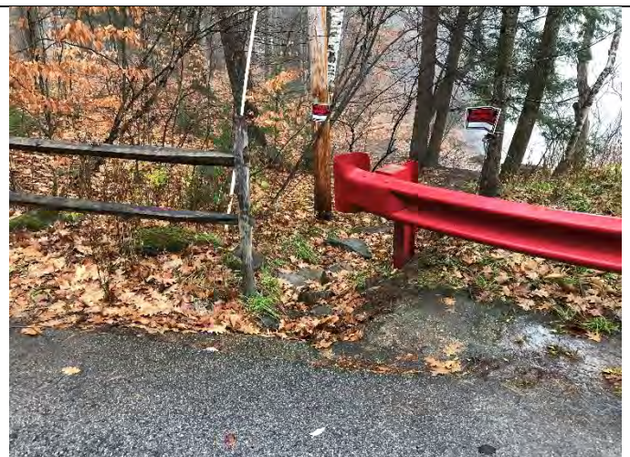
Photo 2: Swale along east side of parking lot that does not receive runoff due to poor site grading
