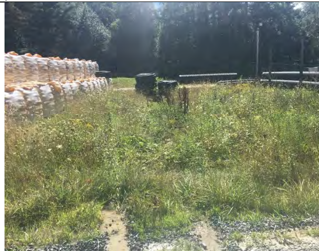
Photo 1: Swale in the middle of the large gravel parking lot. Rill erosion visible in the bottom of the photo.
