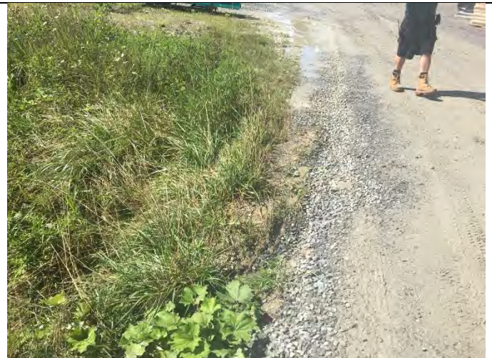
Photo 2: Sheet erosion off gravel parking lot into one of the swales.
