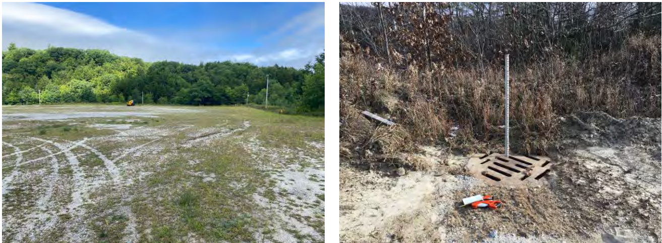
Figure 4: Project LT-04 had the highest score (42 out of 50). The project is located on a Town owned parking lot that is leased by Okemo Mountain Resort (blue lot). A large portion of the gravel parking lot drains to a deep catch basin structure which is directly connected to a stream to the north. Large gully and rill erosion features were observed along concentrated flow paths across the parking area. The opportunity to treat a large volume of water and a very high sediment/nutrient load while on Town property produced the highest score for any of our stormwater master planning projects to date.
