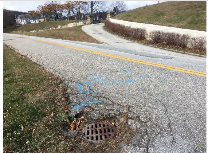
Photo 2: Existing drop inlet, some runoff likely bypasses the DI due to poor grading.
